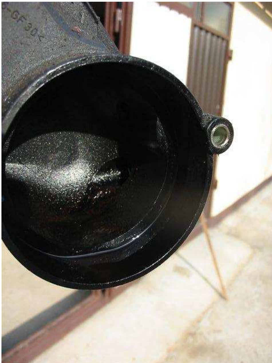
Intake pipe removed. I discovered small oil puddle in the bottom of the pipe.
